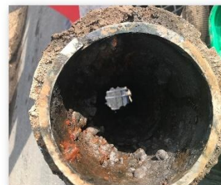
A pipe interior with build-up of suspended solids, corrosion products, and crystallised minerals
