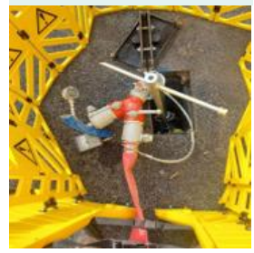
Downstream Hydrant (MH10)
