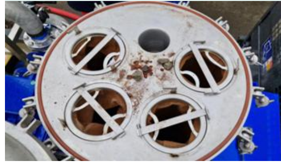
Filter vessel with lid removed showing housing for the 4 fibre filters
